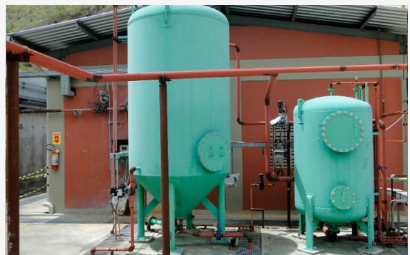
Water treatment plant at Atlantic Nickel
