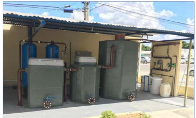
New Water Treatment Plant in União Baiana
