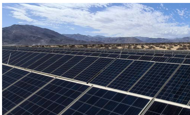
Solar plant at Rosh Pinah
