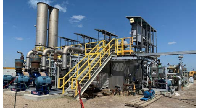
Heating exchange setup at the Milestone Project
